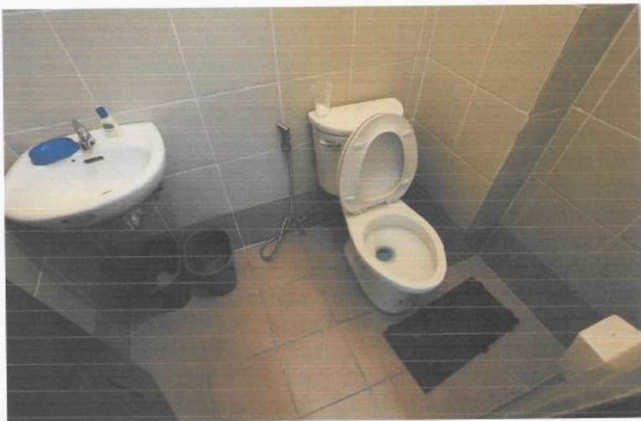
CEA MEDICAL TOILET
